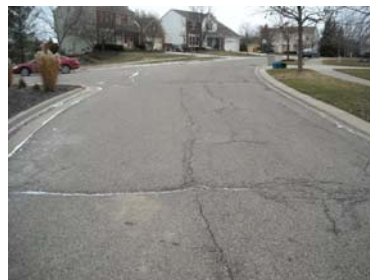
Prior Existing Condition
